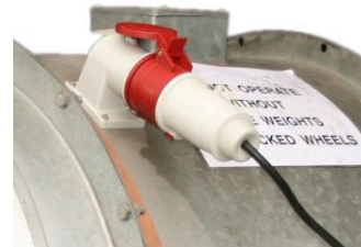
Fig 2. Power Supply 32A 3 Phase
