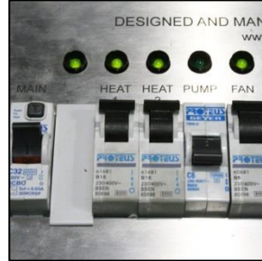
Fig 7. Primary control switches
