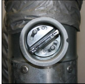
Fig 9. Fog valve partially open
