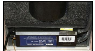
Fig 2. Control unit beneath tube
