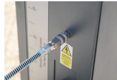
Fig 3. Gas line to Smoke machine
