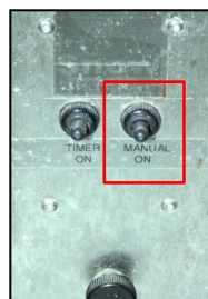
Fig 6. Manual On switch
